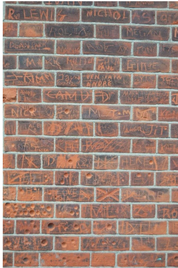
Figure 38 – Graffiti on the wall adjacent to the telephone box
