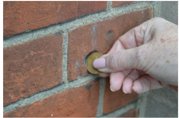
Figure 37 – Soft brickwork with coin
