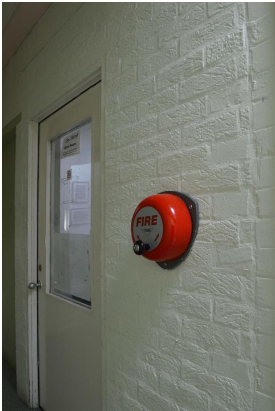
Figure 52 – Corridor with fire alarm
