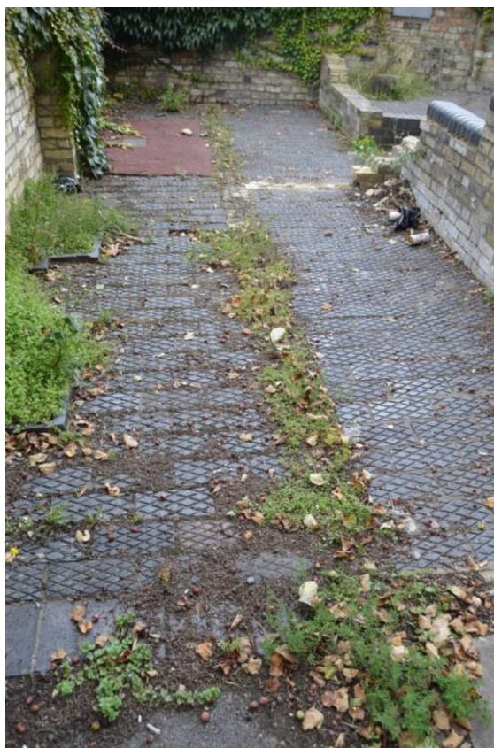
Figure 30 – the old flooring
